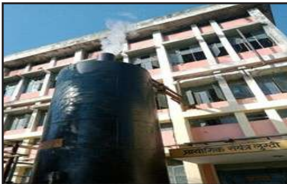
Cooked materials transferred from digester to blowtank
